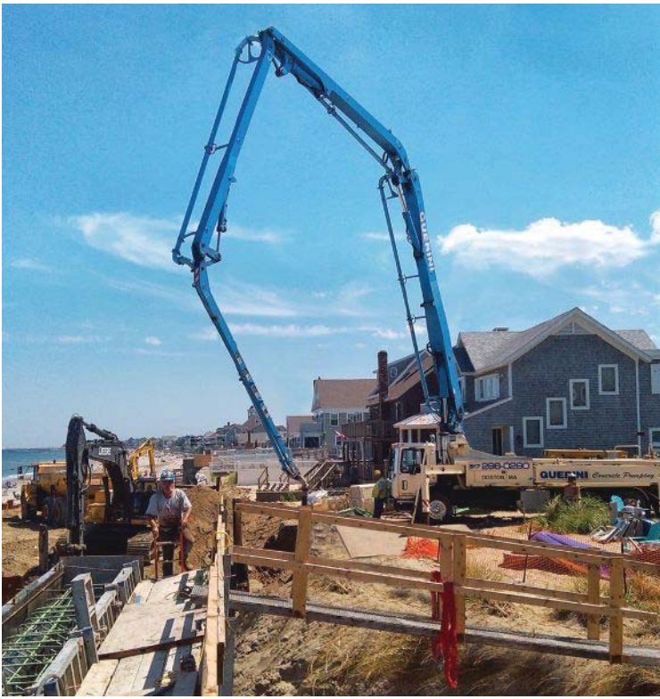
Concrete seawall is reconstructed with use of truck-mounted concrete boom pumps to set up in awkward locations.
