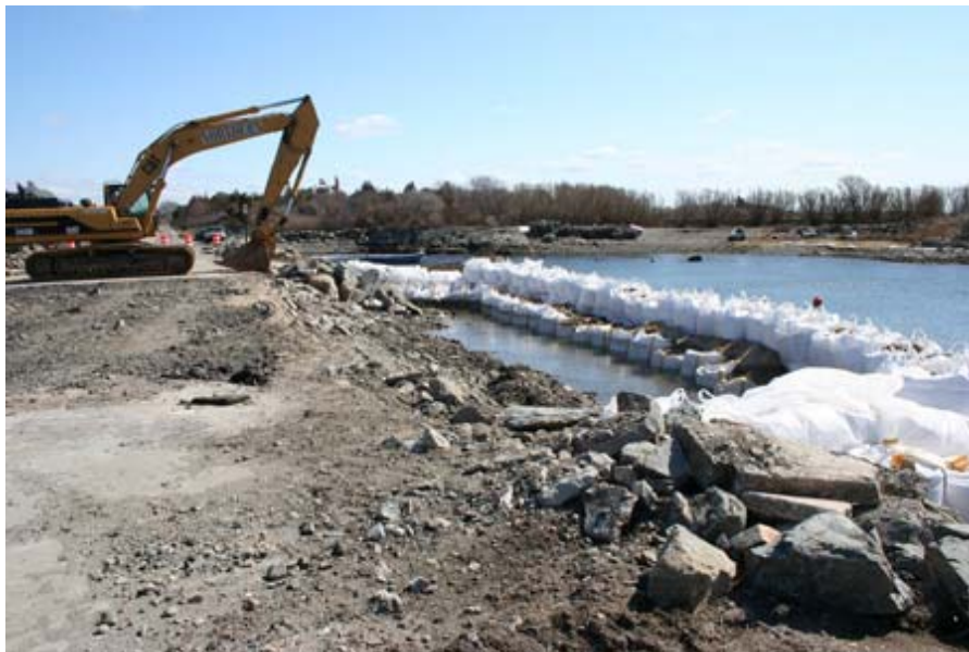
March 24, 2009 - Prep work has occurred at Ocean Drive to prepare for the installation of the three new culverts under the road. The pavement has been removed and temporary dams around the construction area have been created on either side of the road. These areas will be continually pumped free of water to allow for construction.
