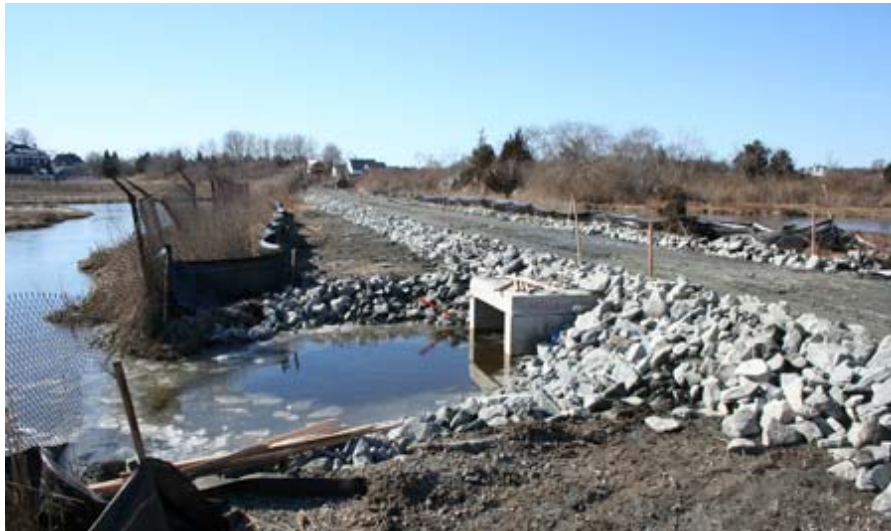
February 25, 2009: The Hazard Rd. culvert has been installed and opened up, and the road subbase has been laid down.
