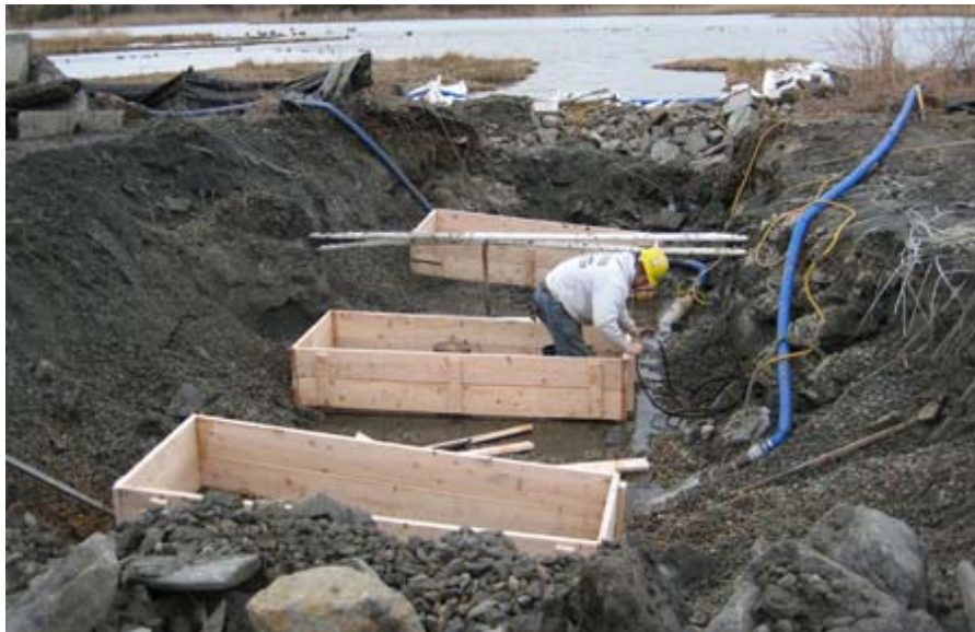
February 2009: Wooden forms are built for the concrete base which will support the culvert on Hazard Rd. The concrete was poured the afternoon of February 12, and the culvert was installed on Friday, February 13.
